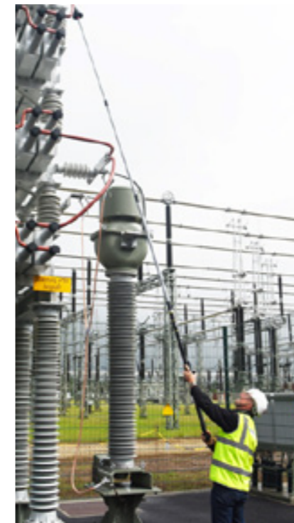
Test at a 36 kV compensation system
